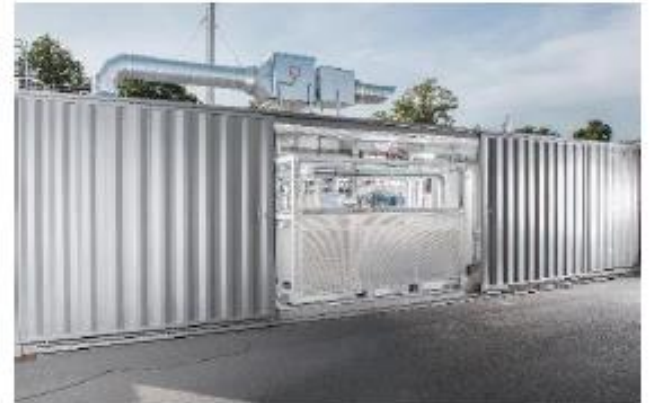
150 kW SOEC unit in Salzgitter, Germany
